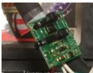
Cable Not Over Sensor Board Oriented Wrong
